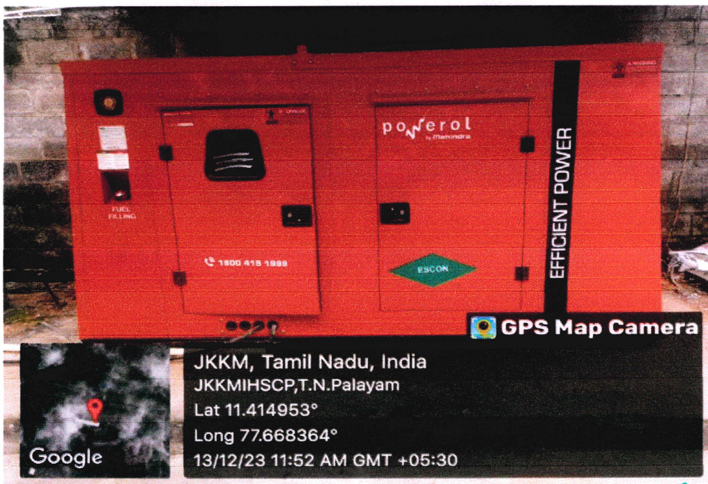
PHOTO OF GENERATOR
