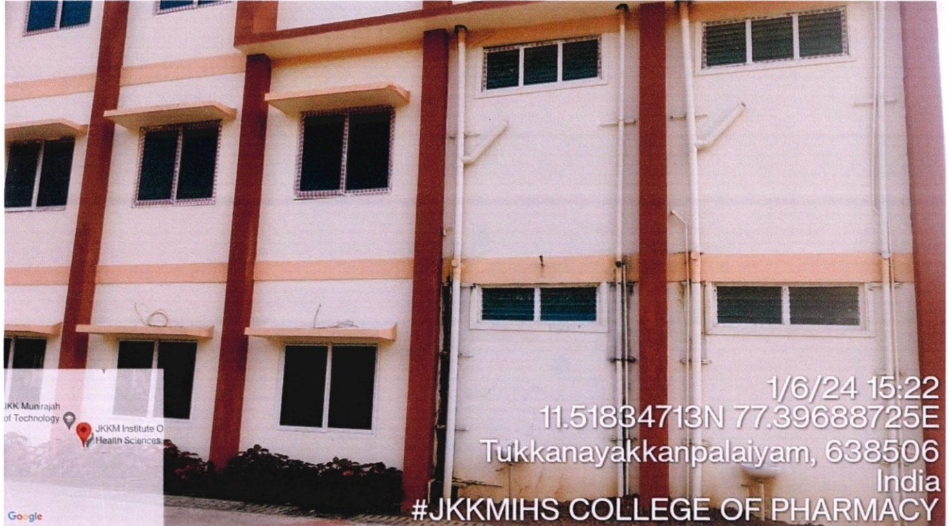
PHOTO OF LIQUID WASTE MANAGEMENT PIPE LINES ON 06.01.2024
